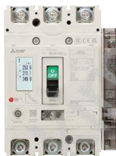
Measuring Display Unit Breaker
